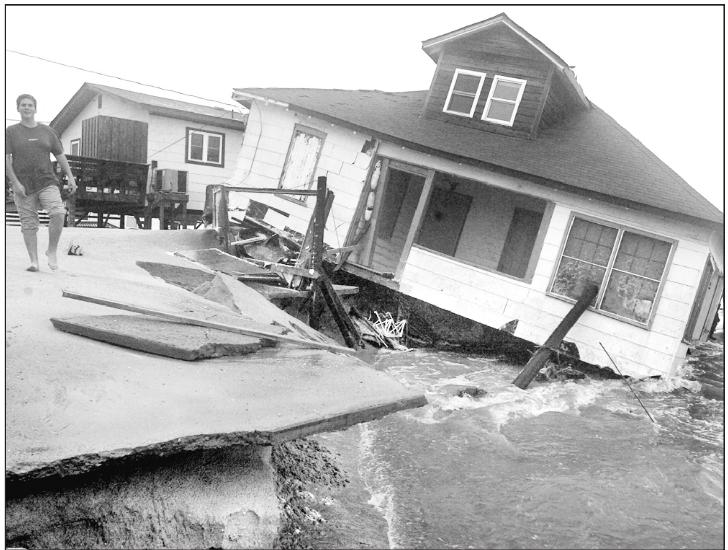
A curious beachgoer emerges after the storm and walks by a beach front home in Kitty Hawk, North Carolina, as it washes out to sea on Thursday in the Outer Banks in North Carolina as a result of Hurricane Isabel. Hurricane Isabel lashed the US East Coast on Thursday killing nine people as winds and floods forced the evacuation of more than 300,000, grounded flights at 19 airports and shut down the US government.
