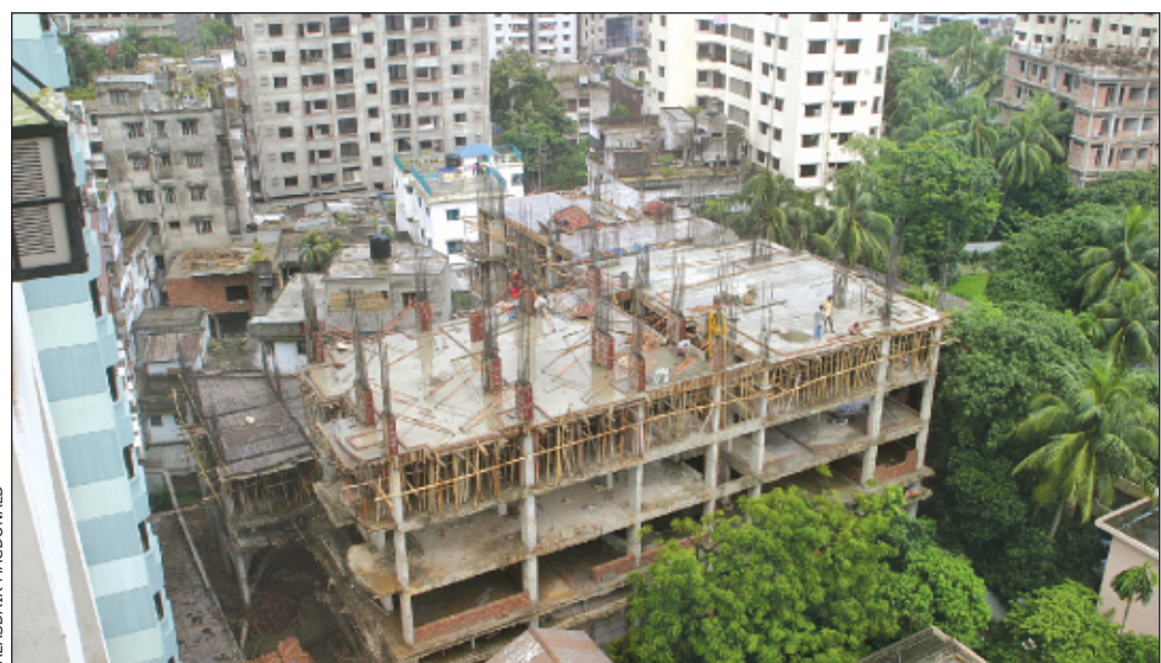
Many of Dhaka's buildings do not conform to the standards set to withstand earthquakes.
