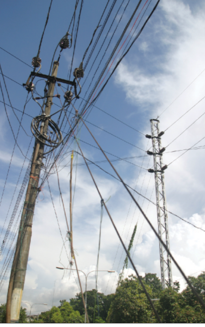
Can DESA poles be used by other service providers without hampering power supply.
