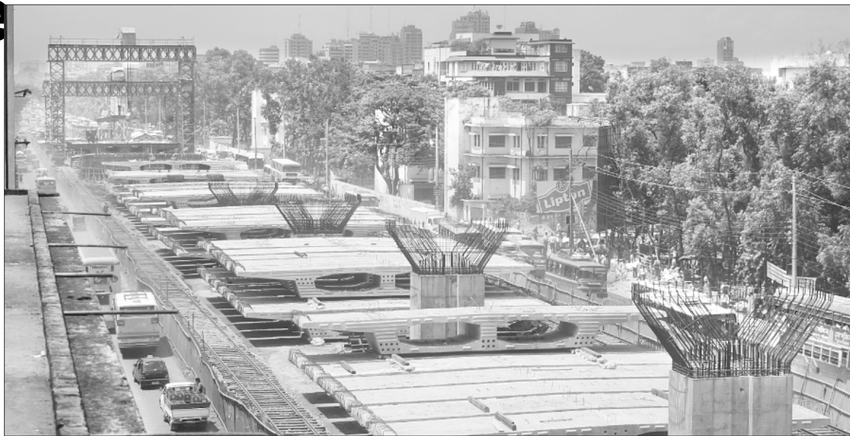
The works of the DUTP include the construction of the Mohakhali fly over, Tongi bypass, and improvement of roads.
