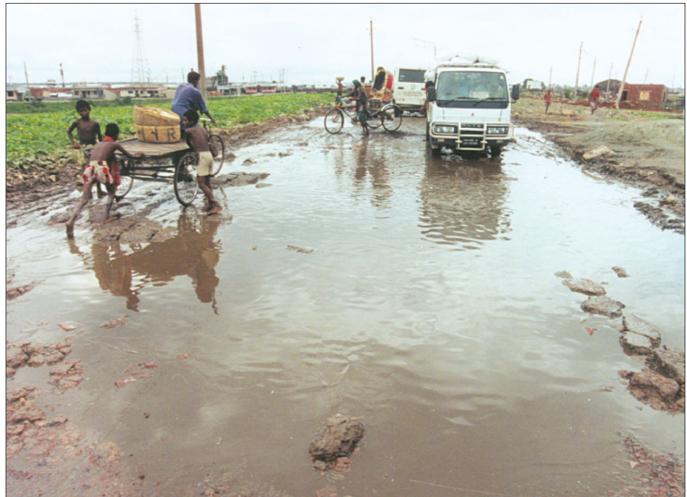
The Gabtali-Kamrangir Char Road, serving as a vital north-south alternative link for the city, is in a rundown condition due to neglect and low quality construction. This picture taken near the Gabtali market yesterday shows the commuters' plight.
