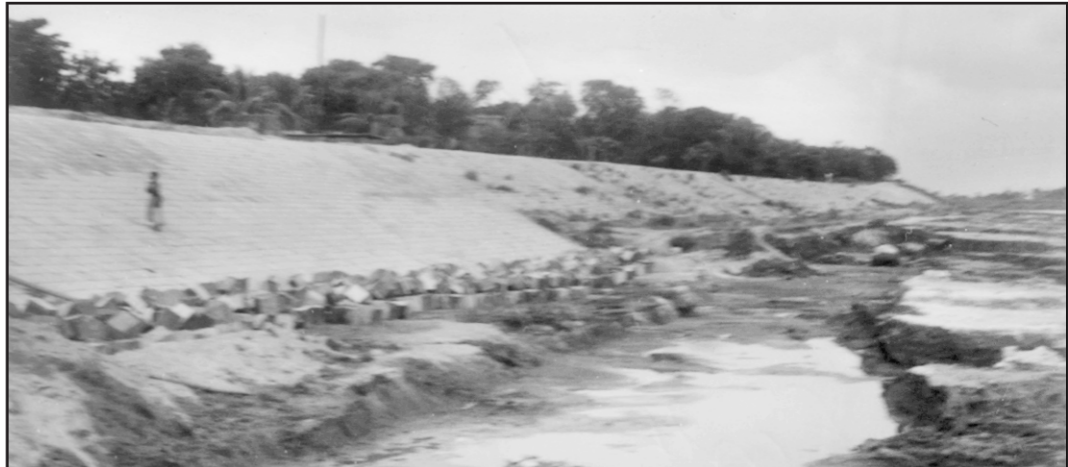
Unabated lifting of earth from the bed of the old Brahmaputra has made the town protection embankment in Mymensingh town vulnerable.
