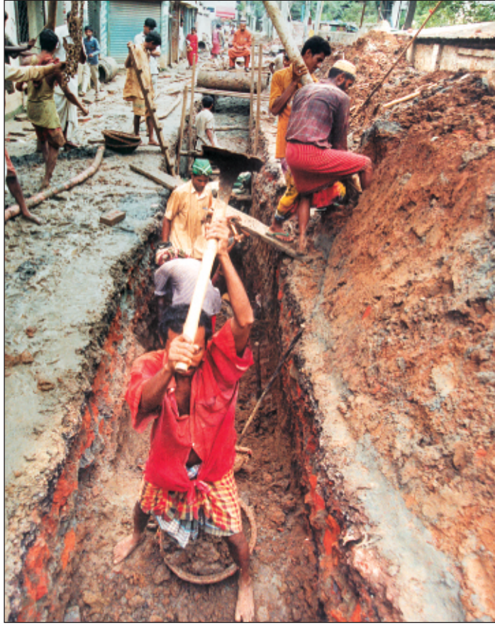
PHOTO: STAR Road digging goes unabated even during the monsoon and more diggings are in the offing with four utility service providers seeking permission to go into the act. Bhooteer Goli, as this picture shows, is one of the worst places to visit now.
