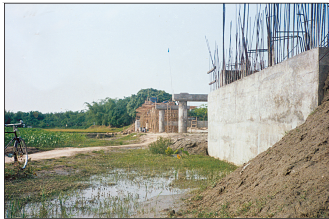
PHOTO: STAR Fund shortage has stalled construction of Megharam bridge on the Ratnai river under Moghalhat union in Lalmonirhat district. The Local Government Engineering Department (LGED) started the work in 2000 during Awami League rule with a budget of Tk 1.06 crore.
