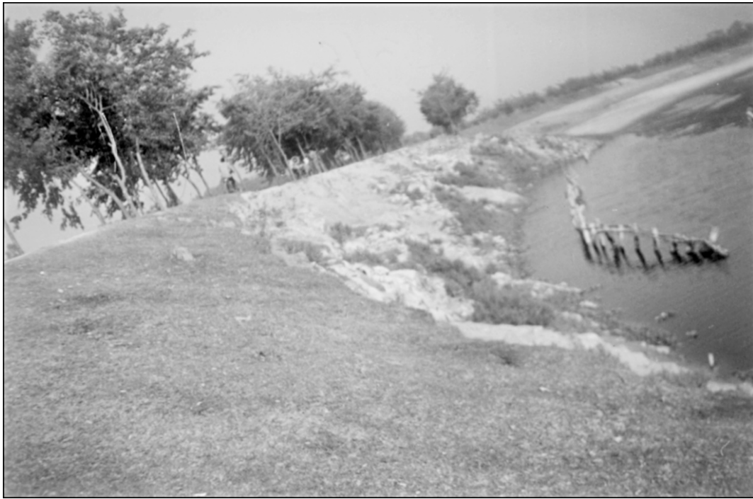
One of the vulnerable points of the Gaibandha Town Protection Embankment. WDB officials fear stretches of the embankment may give in to water pressure and flood the town in the coming monsoon.
