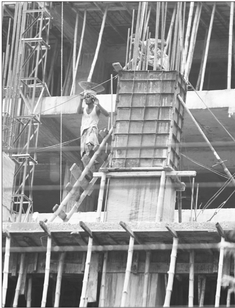
Safety on construction sites lacks supervision or enforcement.
