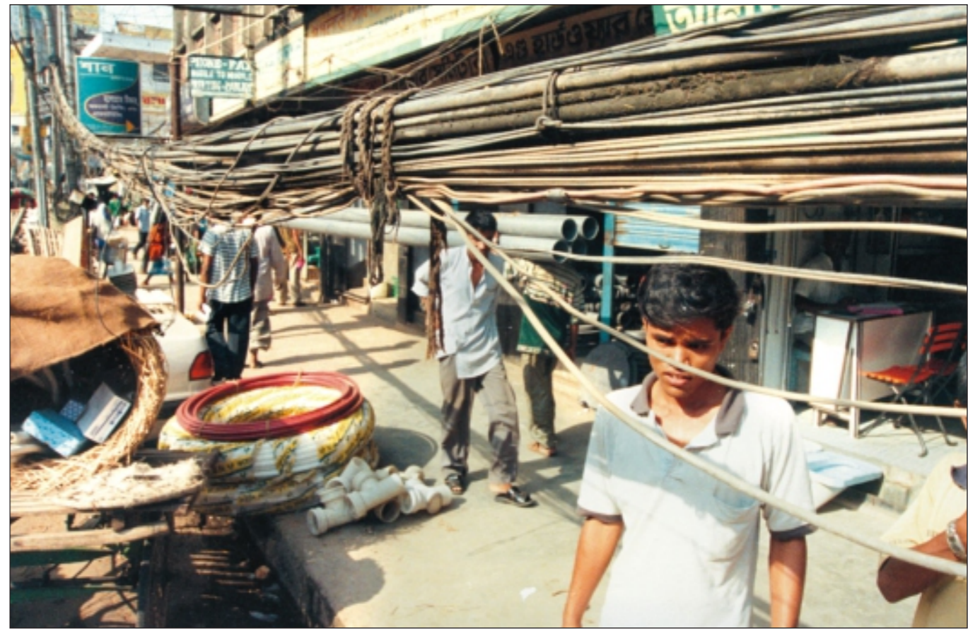
DANGLING DANGER: Passers-by yesterday negotiate a maze of 440-volt power cables and telephone lines hanging just overhead on the North South Road in front of the Saritola school in the old part of the city.
