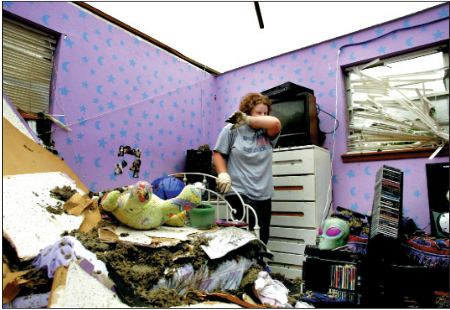
Natalie Stocker, 17, wipes her brow as she tries to salvage what is left of her roofless bedroom on Friday following the previous night's tornado in Moore, Oklahoma, a suburb of Oklahoma City. More than 100 people were injured when the tornado tore through Oklahoma City, flattening homes, hurling automobiles into ditches and snapping power poles and lines.
