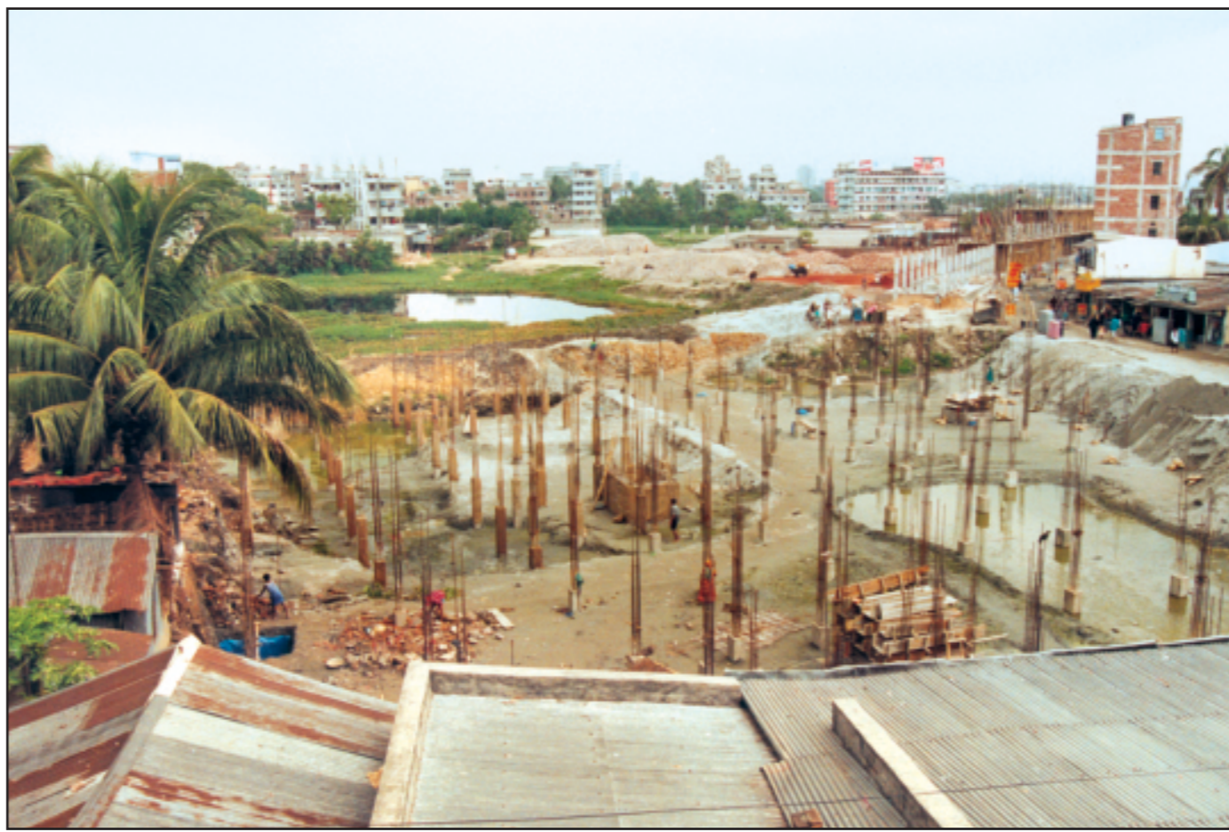
A view of construction of a building on the land allegedly grabbed by Abdul Khaleque, a ruling BNP lawmaker, at Rishipara in Mirpur. Ten families alleged that they lost their land to the construction.
