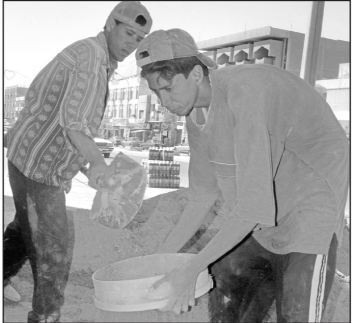
Construction workers mix cement to repair damaged building in Baghdad on Tuesday. Efforts to restore basic services and refashion a government in Iraq inched forward amid warnings by international groups that the war-battered country was still ripe for a humanitarian disaster.
