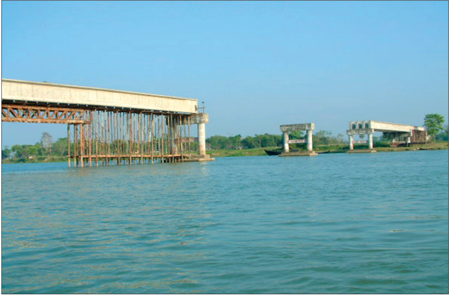
Construction of the bridge over the river Karnaphuli to link Rangunia headquarters and Sarafbhata could not be completed even in seven years. Construction of only two spans could have materialised the dream of the people living on both sides of the bridges.
