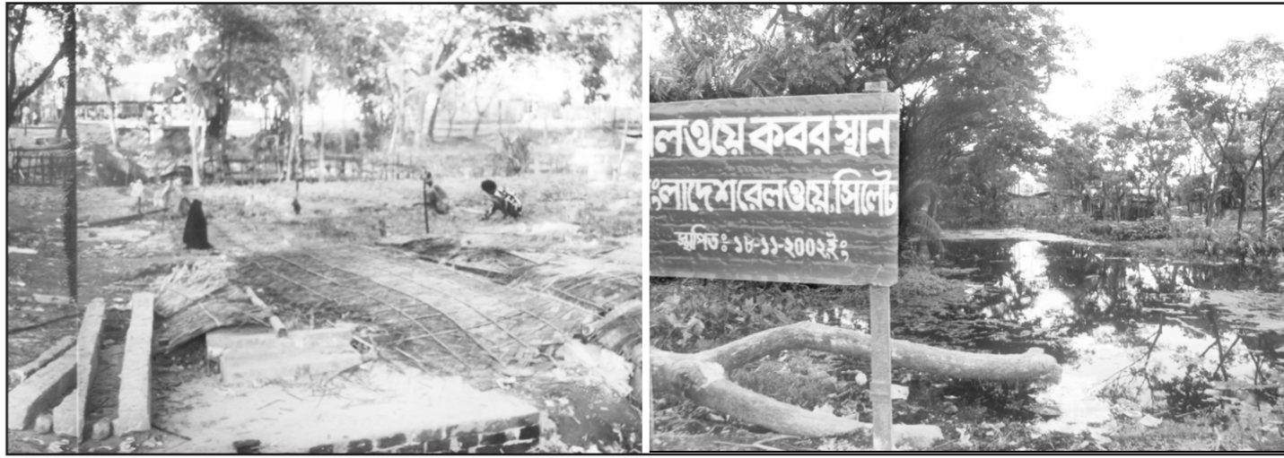
(Left) Some illegal structures on the railway land were demolished in an eviction drive in Sylhet recently, while (right) some railway personnel fixed a signboard in the name of railway graveyard on a vacant land just after the eviction drive.
