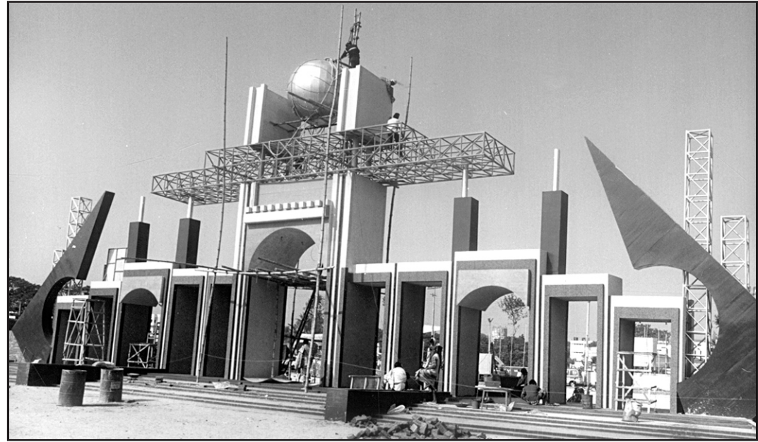
Workers give final touches to main portal at the Dhaka International Trade Fair venue at Sher-e-Bangla Nagar in the city yesterday. The ninth version of the month-long annual event begins today.
