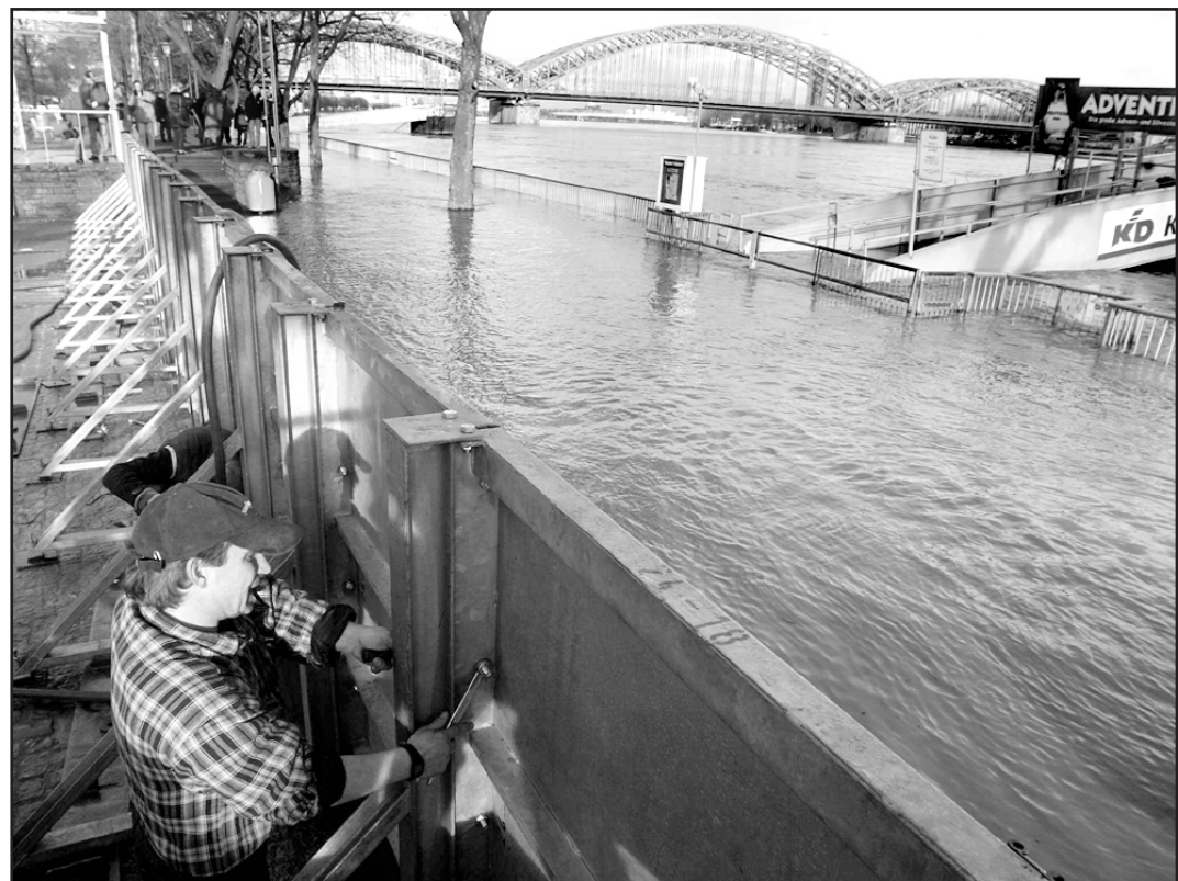
A worker installs a water-barrier on the riverside walk of river Rhine in Cologne, Germany on Friday. Incessant rain has swelled watercourses in Bavaria and Cologne.
