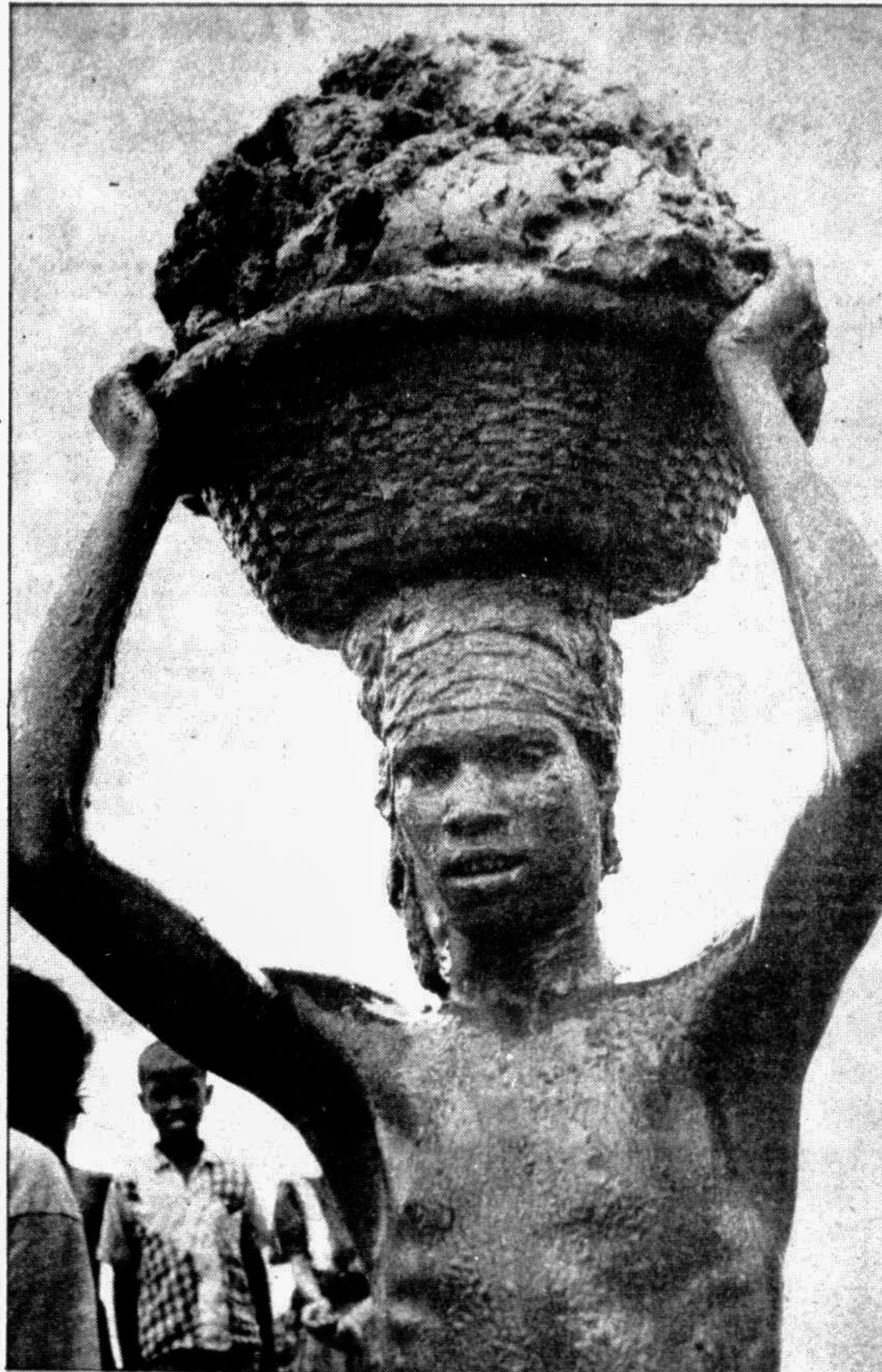
STRUGGLE FOR SURVIVAL: A day's hard labour at a road construction site under the Food for Works Programme at a village in Comilla gets this young man just enough wheat for a family of four that he maintains. Tomorrow, for him, is uncertain. — Star photo
