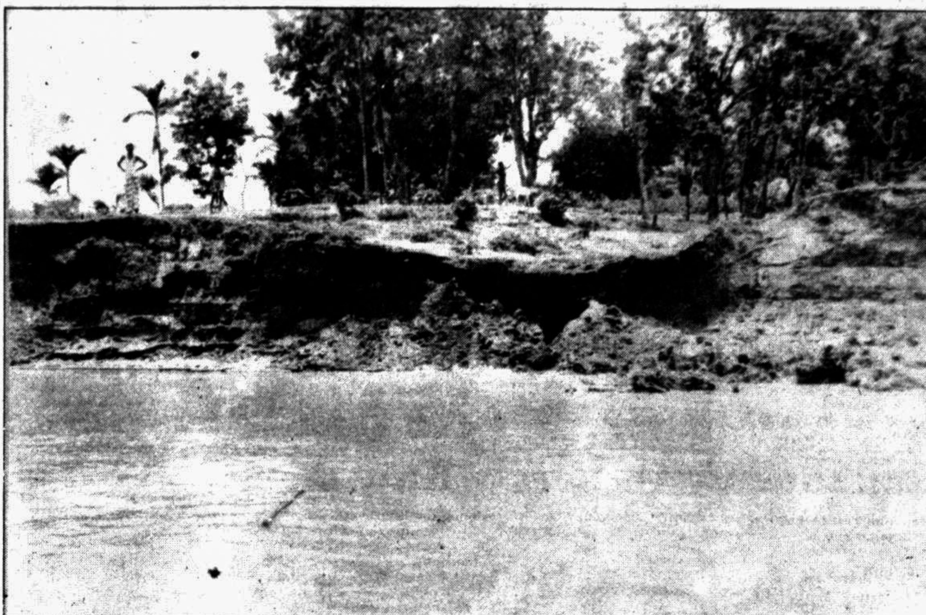
RANGPUR : A view of the erosion of the river Teesta at Gongachara.
